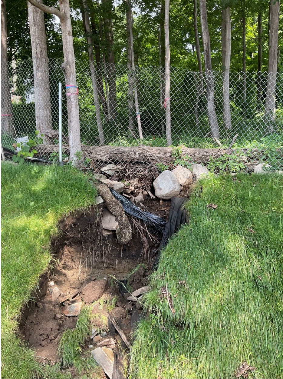
Photo of area of erosion taken by Staff on July 22, 2026
